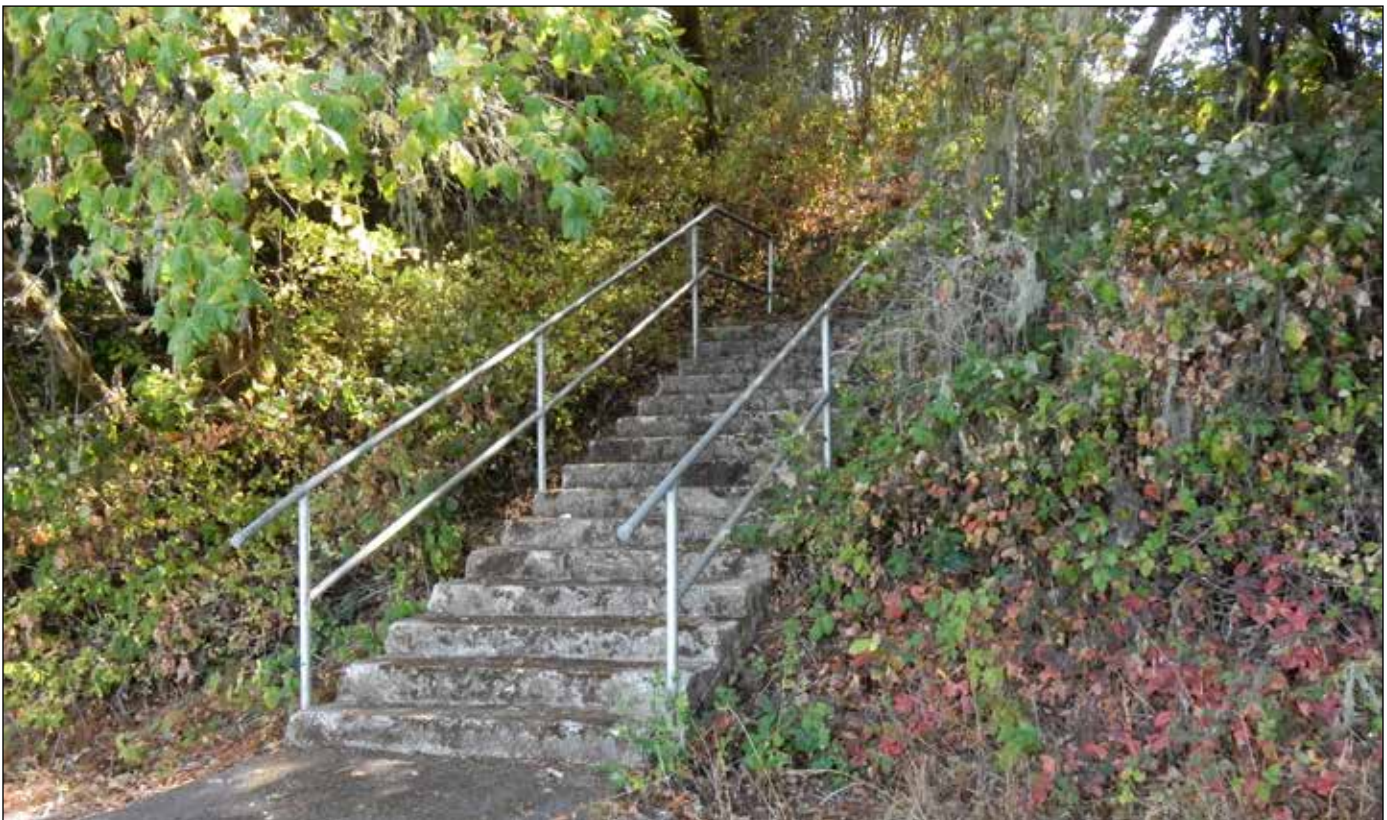
Deteriorating Stairway at Perkins Peninsula County Park
