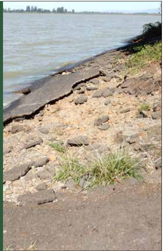
Deteriorating Revetment at Perkins Peninsula County Park
